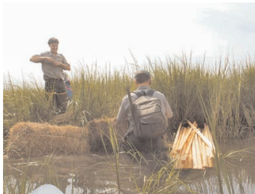
Figure 2. Before spraying sand on the Big Egg Marsh restoration site, 240 hay bales were staked across the drainages to contain the runoff of silt and organics.
