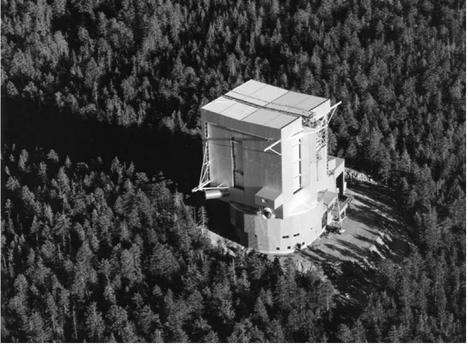
Figure 2. An aerial view of the LBT (Large Binocular Telescope) enclosure erected on Mount Graham during December 1999. As of April 2004, construction was continuing on the telescope itself. Photo by Stephen Criswell courtesy of Large Binocular Telescope Project.
