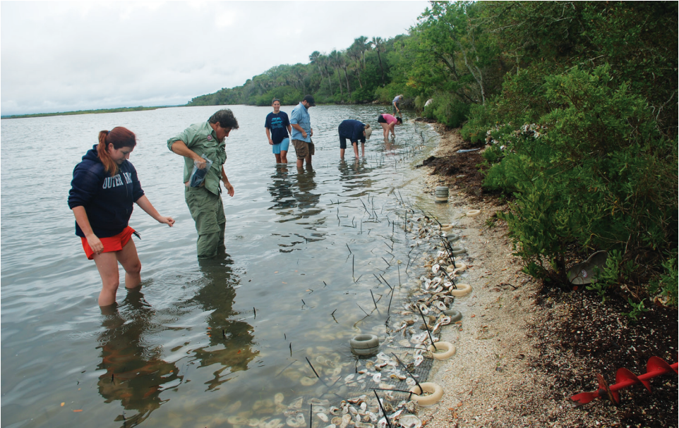
Figure 1. Workers install oyster shell mats as part of the living shoreline project in Mosquito Lagoon at Canaveral National Seashore. M. Schwadron/National Park Service photo.
